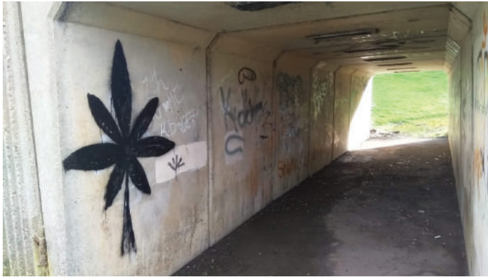
Areas like this show decay and make people feel unsafe. Labour Councillors want to target areas like this and urge regeneration - improving ASB and perceptions of safety.
